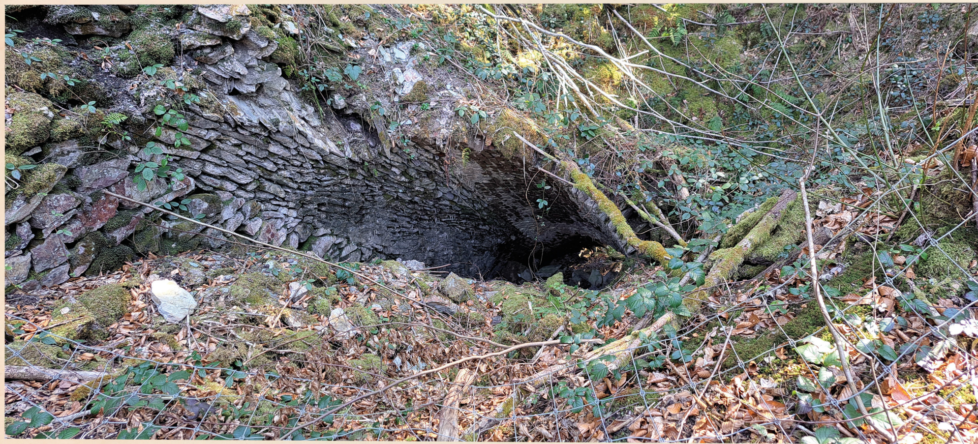
Collapsed entrance of the Notre-Dame slate mine
